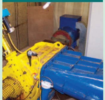
The 90Kw crossflow turbine and generator
