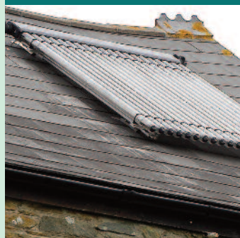
Solar thermal panels
