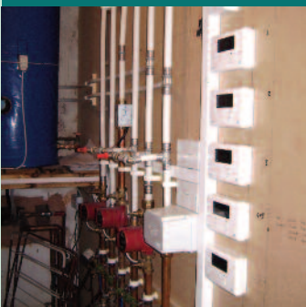
Heating and hot water controls
