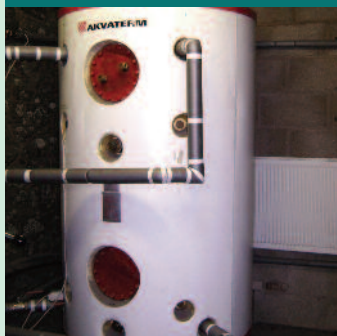
Typical accumulator tank
