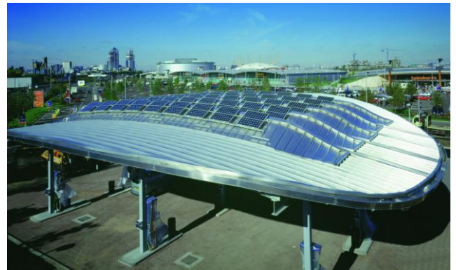
FIGURE 2: LARGE-SCALE PV INSTALLATION (SOURCE – SOLAR CENTURY)
