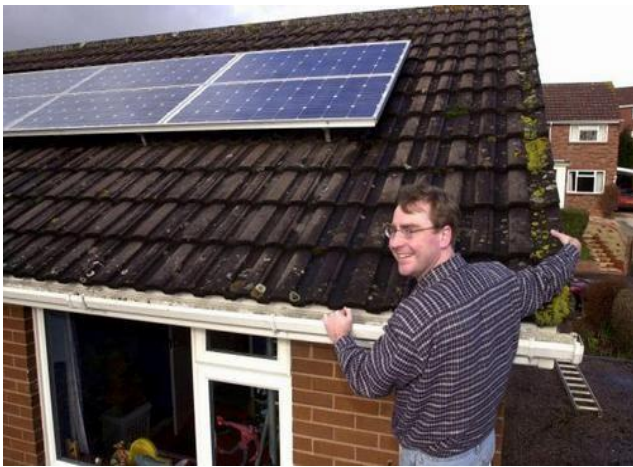
FIGURE 3: DOMESTIC SOLAR PV (SOURCE - SOLAR CENTURY)
