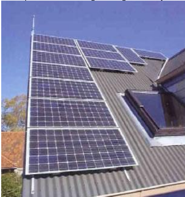
FIGURE 1: ROOF MOUNTED SOLAR INSTALLATION
